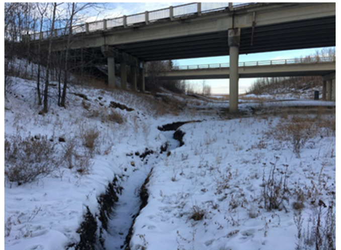
Figure 5: Looking north, scour at mine haul road
