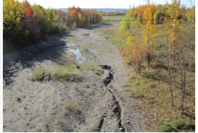
Figure 3: Looking south, drainage path & scour
