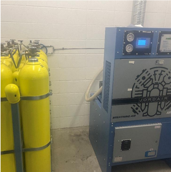
SCBA Fill Station
