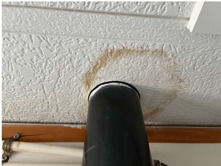
PICTURE 10 – SIGNS OF WATER DAMAGE IN CEILING
