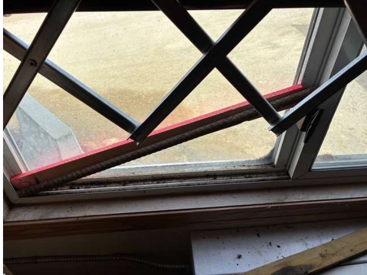
PICTURE 11 – INADEQUATE SECURITY MEASURES
