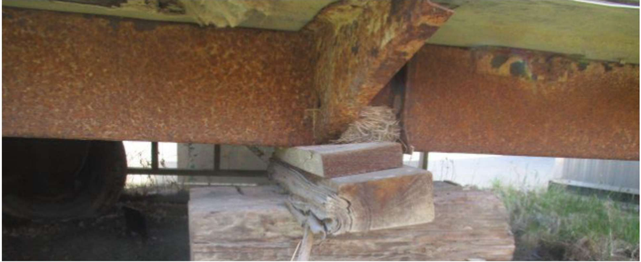
PICTURE 5 – SIGNIFICANT WEAR ON STRUCTURAL FRAME
