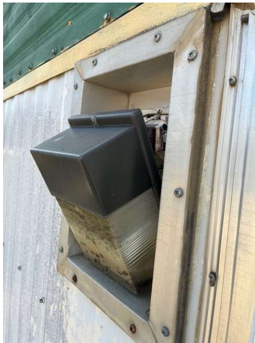
PICTURE 6 – LIGHTING SEPARATED FROM JUNCTION BOX
