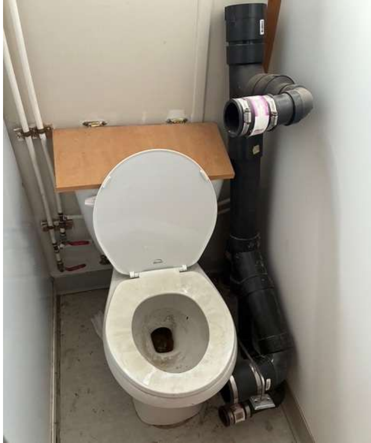
PICTURE 9 – PLUMBING OUT OF SERVICE
