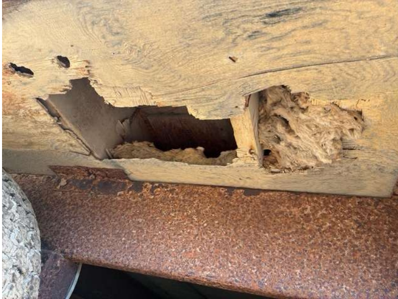
PICTURE 7 – HOLES IN SUBFLOOR, REMNANTS OF INFESTATION
