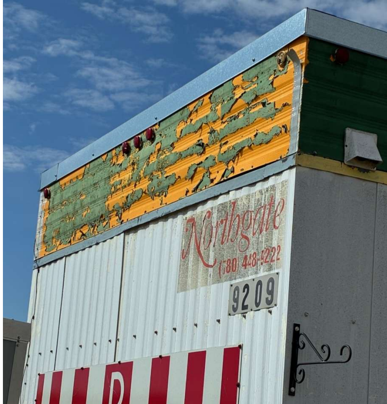
PICTURE 3 – SIDING IN DISREPAIR
