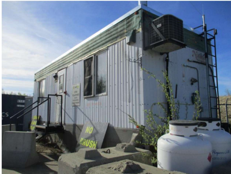
PICTURE 1 – SIDING IN DISREPAIR
