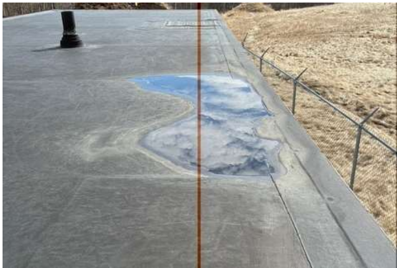
PICTURE 8 – STANDING WATER ON ROOF
