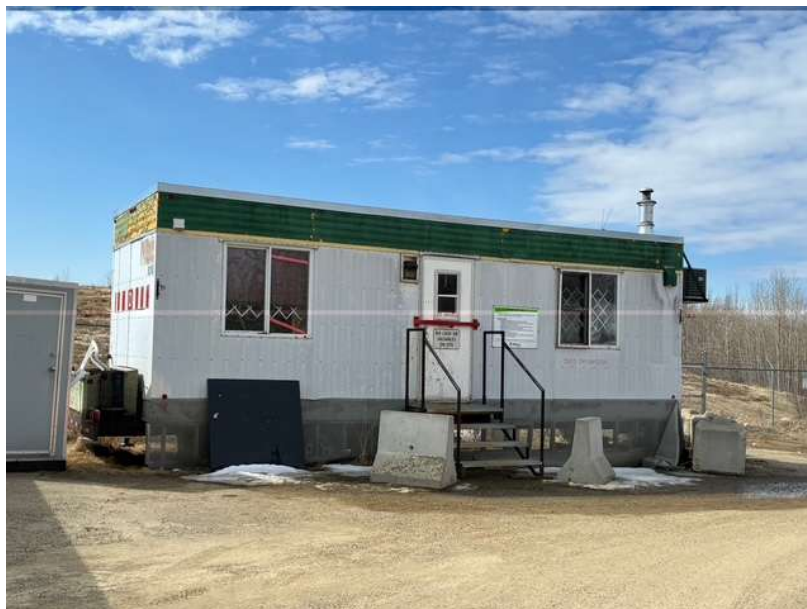
PICTURE 2 – MISSING SKIRTING
