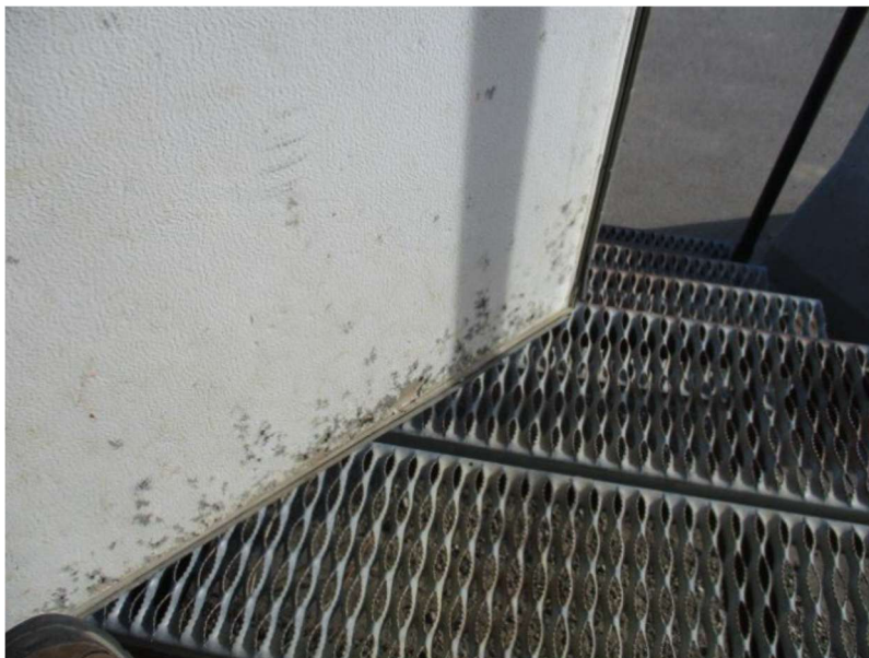
PICTURE 4 – DAMAGE TO DOORWAYS
